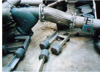
Fig. 9-1 Damage to pipe connection due to footing independent displacement
