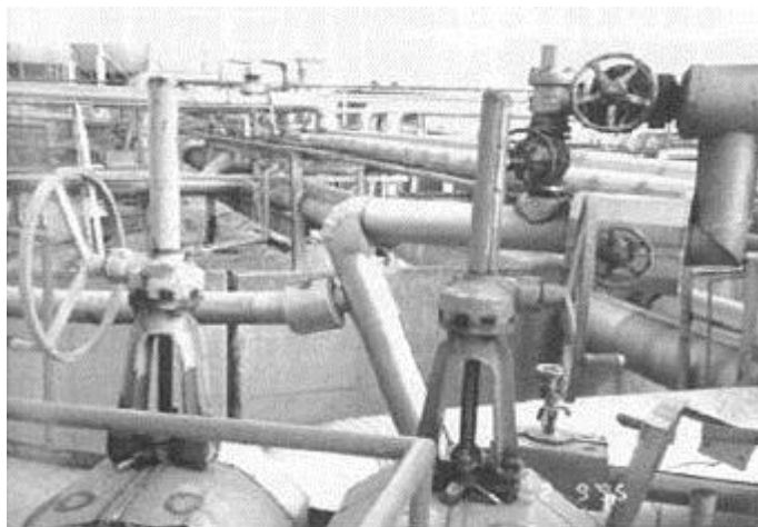
Figure 5-1 Damages in pipes with small diameter
