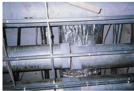
Fig. 9-3 Damage to piping of water cooling system (Due to lateral seismic force, the welded part of pipe has damaged)
