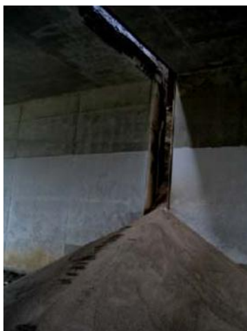
Fig 10-2. The gap in the culvert with square cross section due to earthquake
