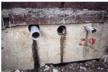
Fig. 9-4 Piping in the building inlet
