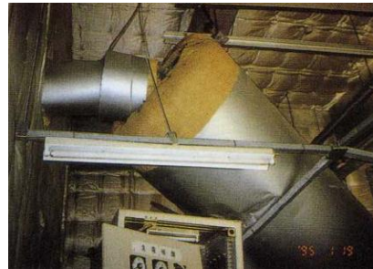
Fig. 9-5 Damage to sound-proof element
