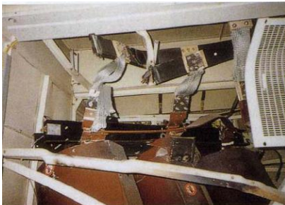
Fig. 9-8 Damage to transformer and its elements
