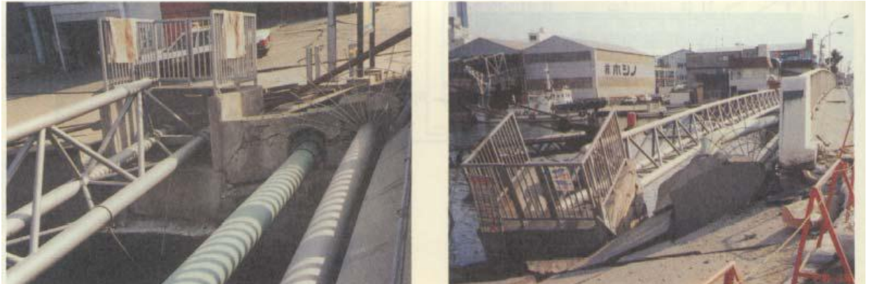
Figure 7-2 Damage to pipeline due to failure of bridge in spread liquefaction
