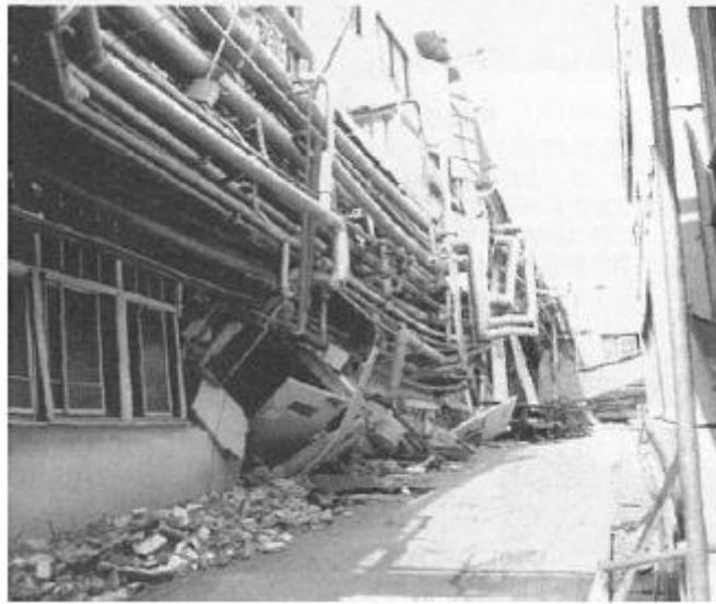
Figure 5-4 Damage to piping system due to damage to building
