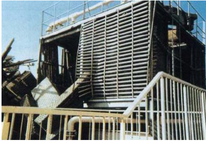
Fig. 9-2 Damage to cooling tower. No slide is reported due to existence of fillers (structures).
