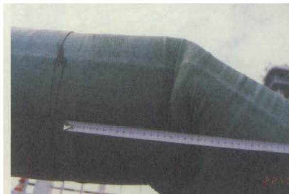
Figure 7-1 Cracks and buckling in bent pipe
